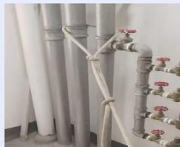
Metal drainage pipe
